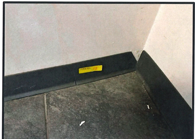
Photo #: 12 Material #: 12 Non-ACM Subject: View of 4" Grey Cove Base w/ Adhesive. Located in the conference room.
