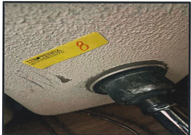
Photo #: 8 Material #: 8 Non-ACM Subject: View of White Sink Undercoat. Located the kitchen and nursery.
