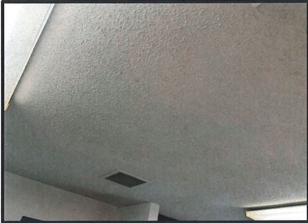
Photo #: 1 Material #: 1 Non-ACM Subject: View of Textured Ceilings. Located on ceilings throughout.
