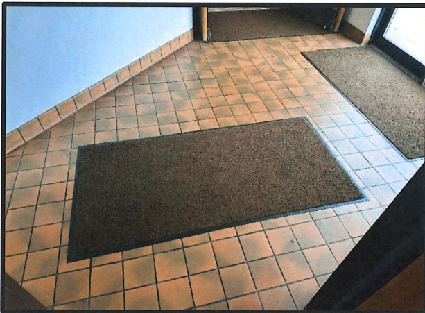
Photo #: 9 Material #: 9 PACM Subject: Presumed Asbestos-containing Terra cotta Floor Tile. Located in entries.
