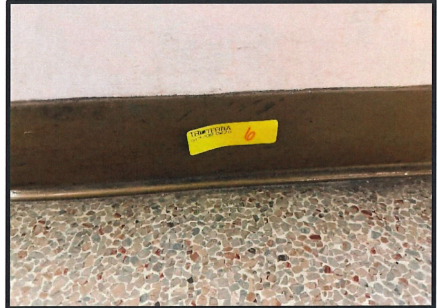
Photo #:6 Material #:6 Non-ACM Subject: View of 4" Brown Cove Base w/ Adhesive. Located various rooms. See table.
