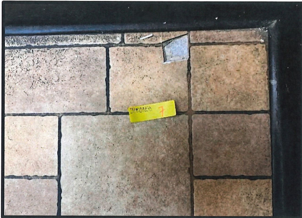
Photo #: 7 Material #:7 Non-ACM Subject: View of Tan Sheet Flooring w/ Brick Design. Located in various rooms. See table.
