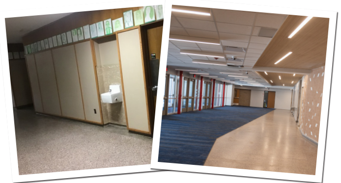
Before and after photos of the atrium at Everett. These are just a sample of the work, but the improvements are significant.
