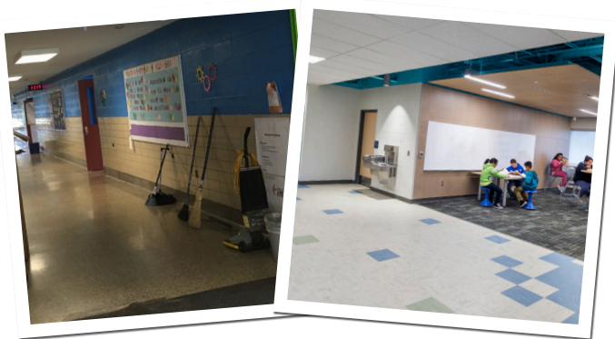
The left photo shows a dark dingy hallway at Pattengill, the right shows the renovated space post 2016 bond work.
