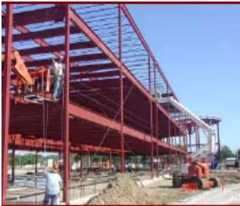
Structural steel in place at the new Pattengill Middle School. The photo shows the three story tall classroom area.
