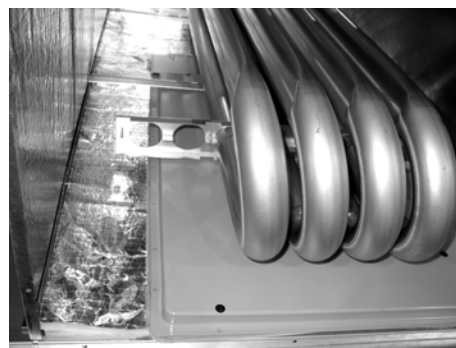
Figure 19: Discharge Panel In Place
