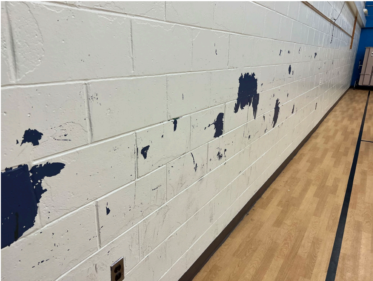
Figure 2: Peeling paint on East wall Multi-Purpose Room
