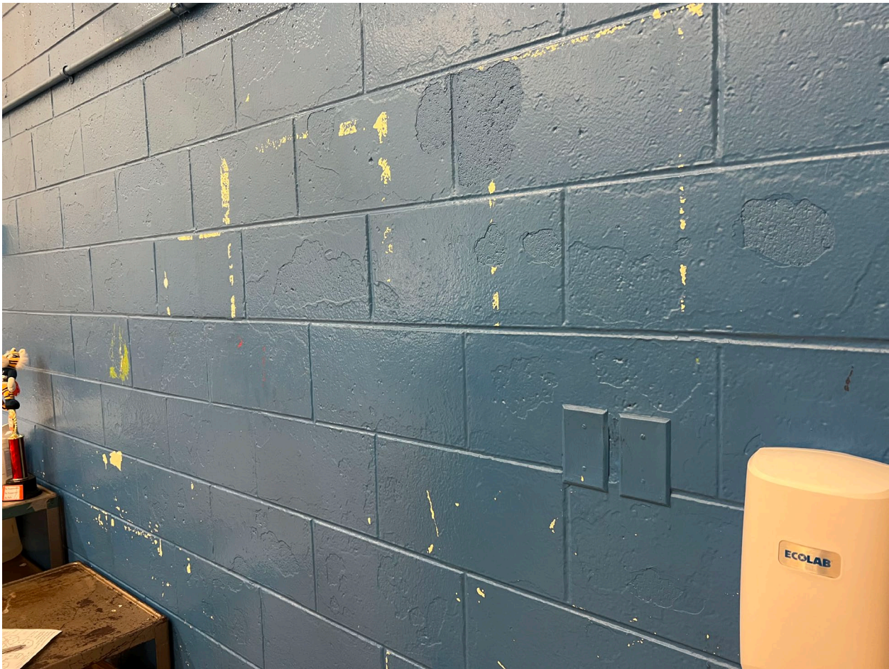
Figure 3: Peeling paint on North wall Multi-Purpose Room
